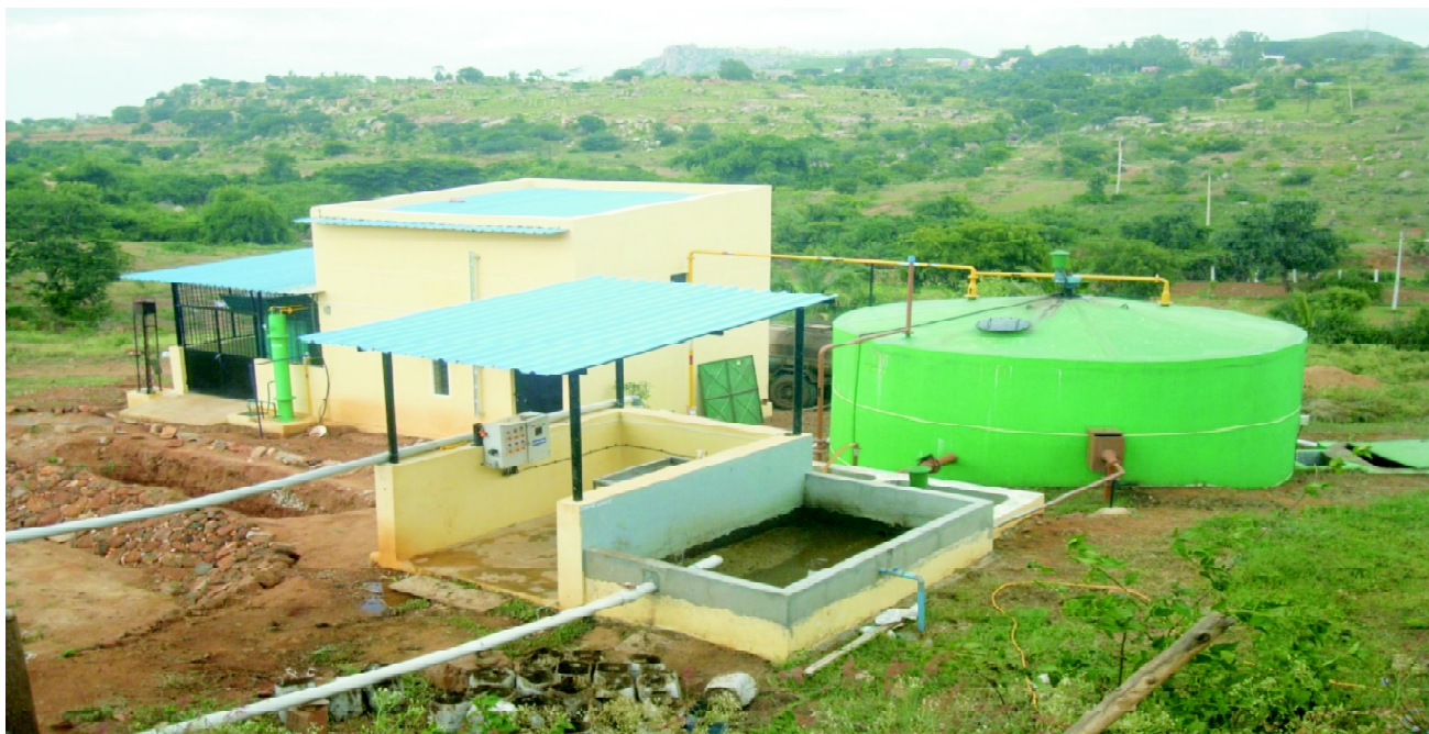
Rashthrothana Goshala-Biogas Power Plant
