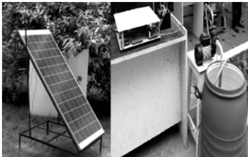
Figure 13: Hardware setup of Induction Motor Pumping
