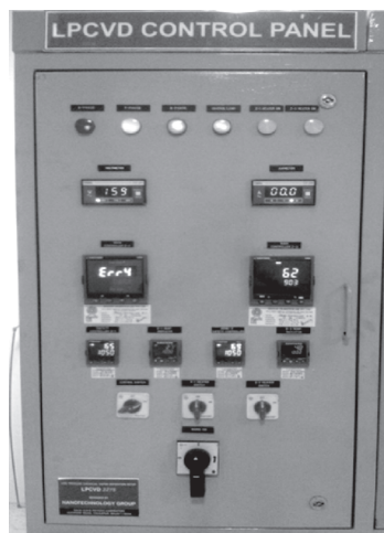
Figure 2: LPCVD Control Panel
