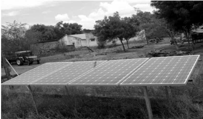
Figure 2: PV panels as distributed generation
