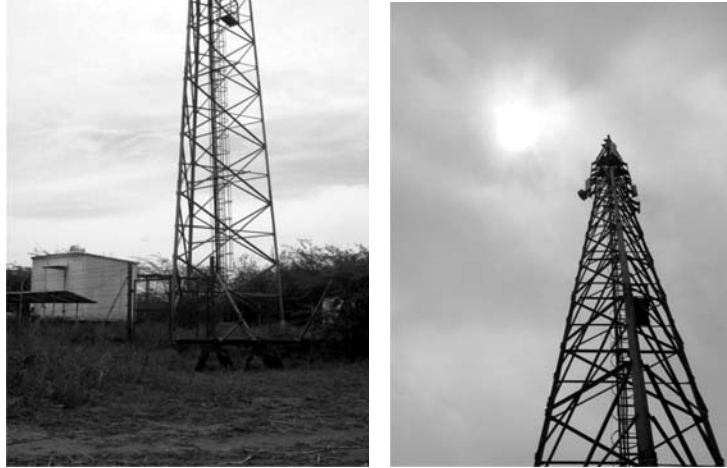
Figure 1: BSNL Tower in Silarpatti village
