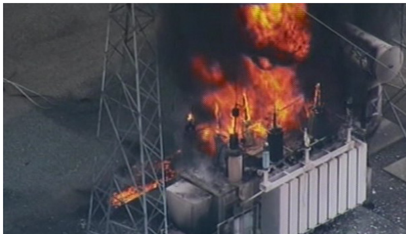
Figure 2: Fire due to mineral oil from a high voltage transformer ( http://www.nbcrightnow.com/story/14924340/ )
