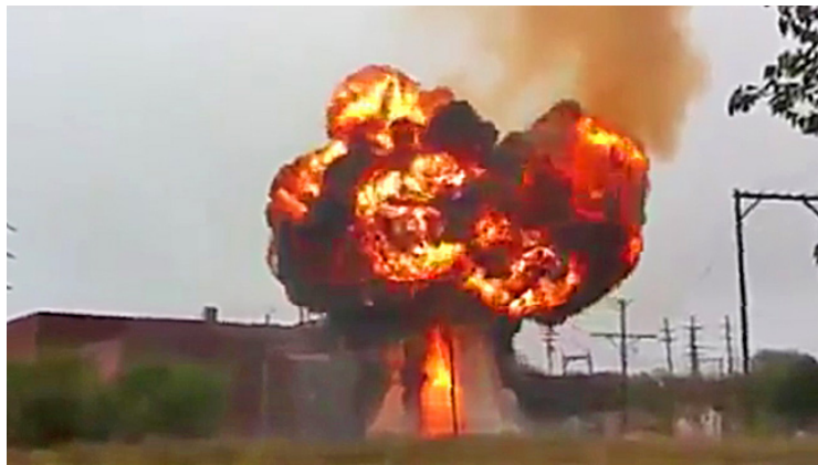
Figure 5: Transformer explosions ( http://video.news.com.au/v/75639/ )
