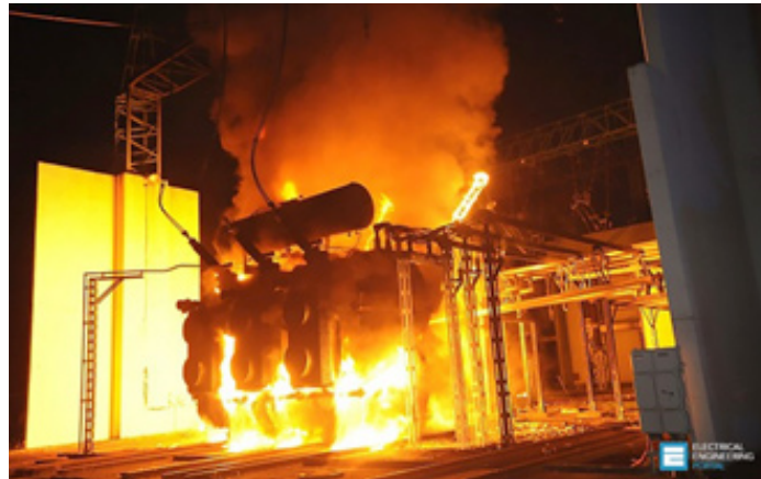
Figure 7: Firewalls containing the transformer fire ( http://electrical-engineering-portal.com/substation-fire-protection )
