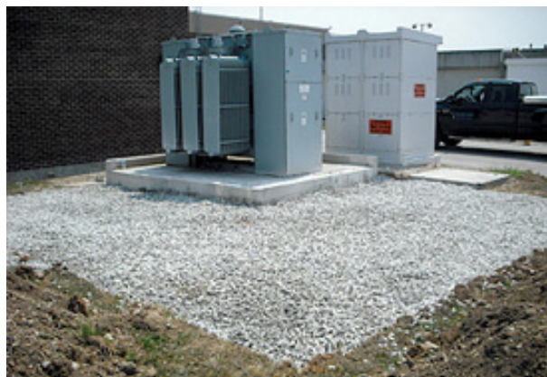
Figure 6: Transformer oil containment ( http://www.transformer-oil-containment.com/ )
