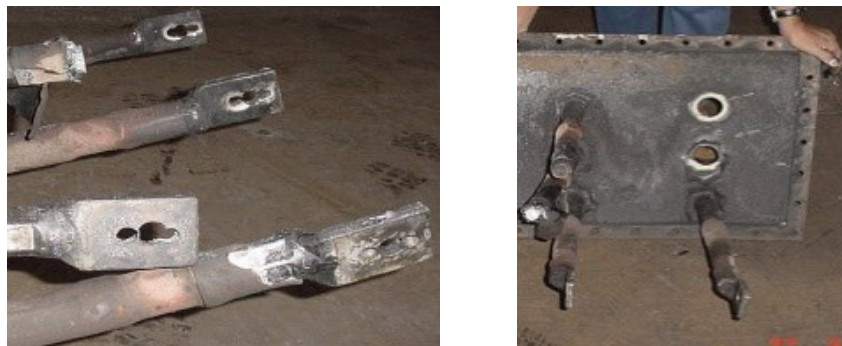
Figure 3: Bolt holes of the lug of the transformer destroyed by fire (www.lankaweb.com)
