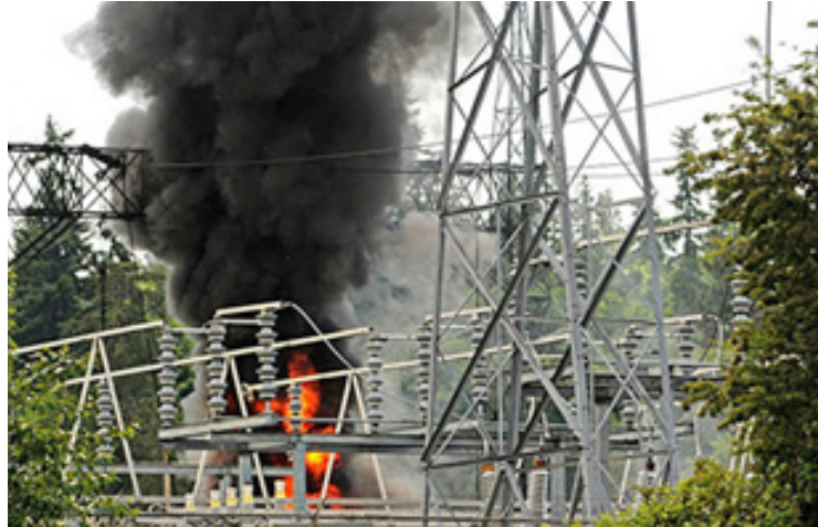
Figure 4: Overhead structure fire that cause metal structures to sag and collapse. ( http://electrical-engineering-portal.com/arriving-at-the-scene-of-a-power-substation-fire )
