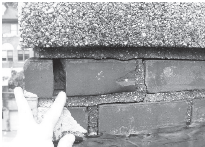
Figure 4: Crack Resulted due to improper construction
