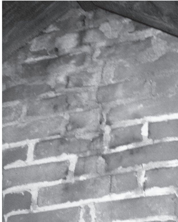
Figure 5: Cracks caused due to seepage of water
