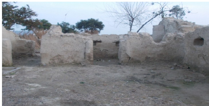
Figure 2: A house destroyed by floods in Bahraich
