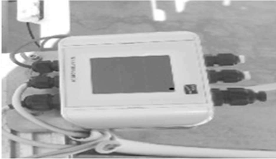
Figure 2: Solar sensor box
