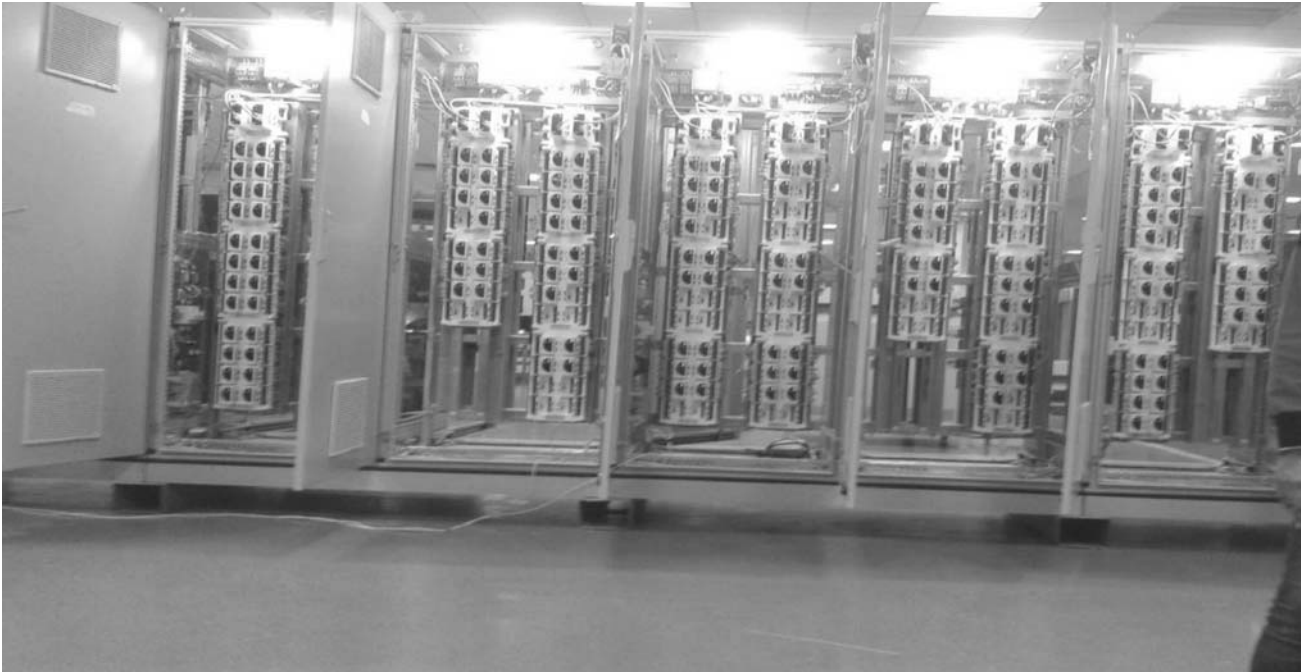
Fig. 5. I/O ring Network into the panels for controlling signals of a control system.
